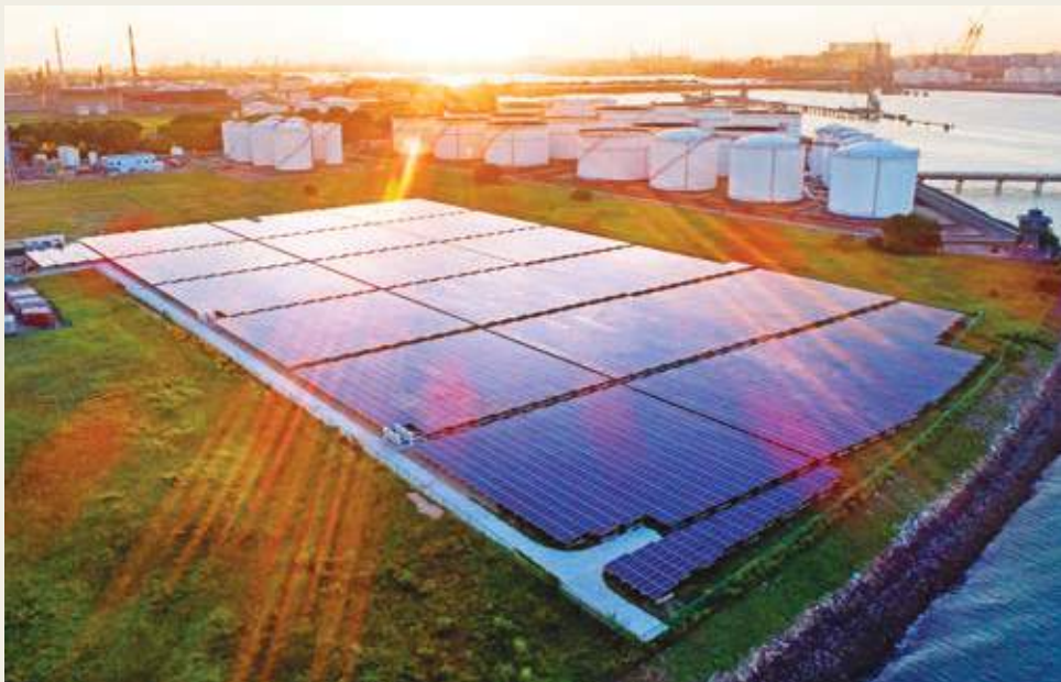
SolarLand at Jurong Island utilises vacant land to generate clean energy Photo courtesy of JTC
